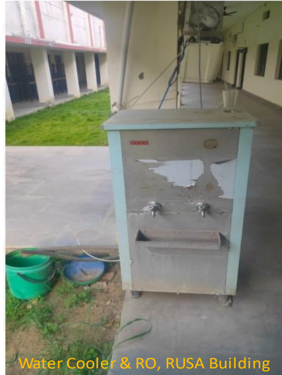
Water Cooler & RO, Main Building
